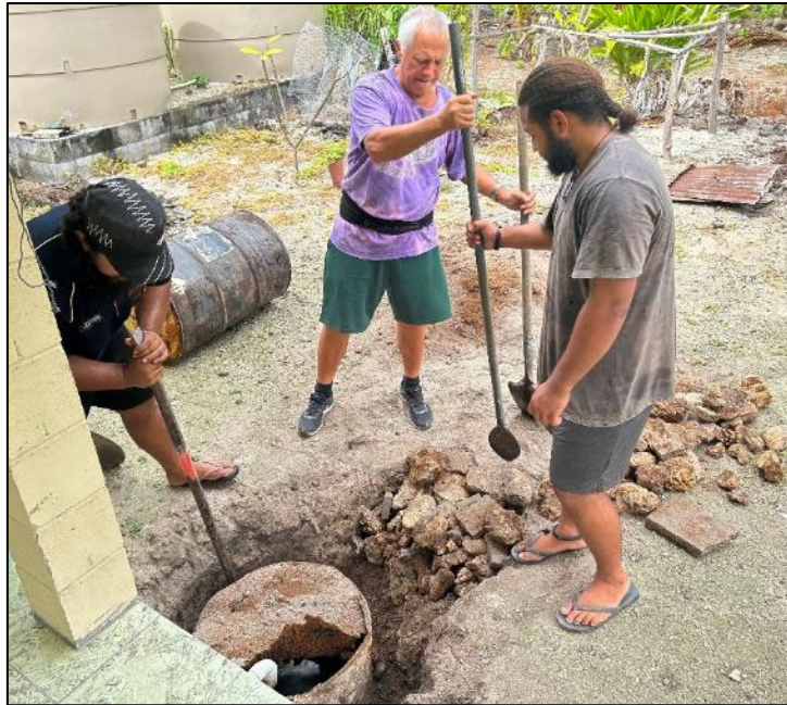
Figure 2.1.3: Community members addressing containment of waste water from a residential building
