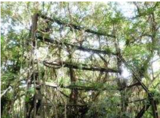
Plate 2: The remains of a phosphate storage facility from the German mining era
