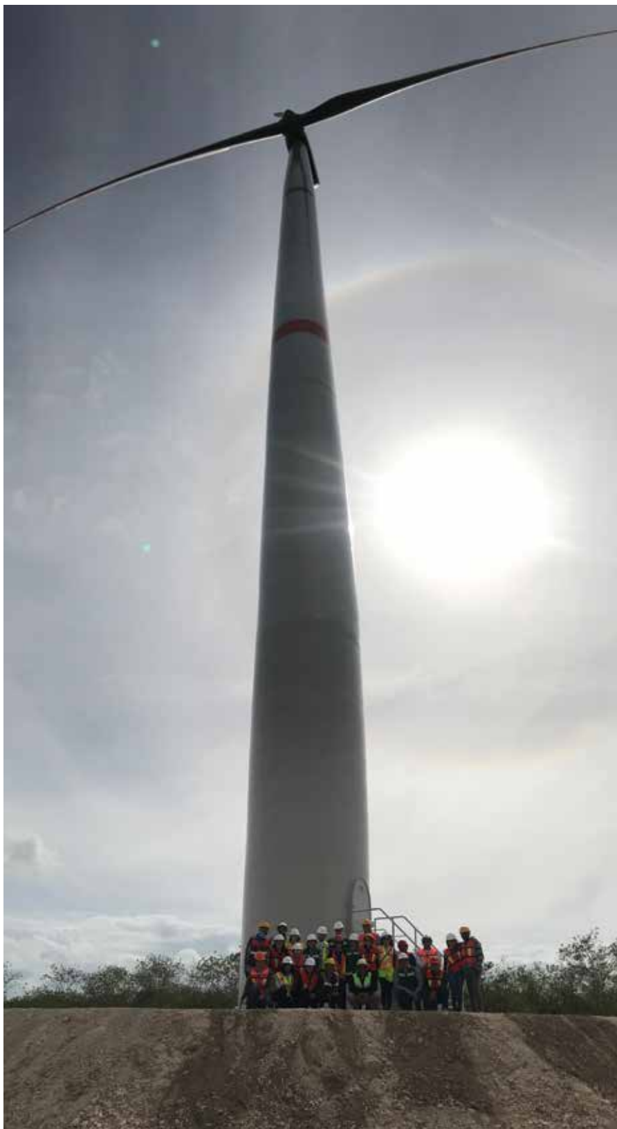
Dzilam Bravo Wind Farm currently has 28 330-foot tall wind turbines under construction and will provide renewable energy to approximately 32,000 homes in the area.
